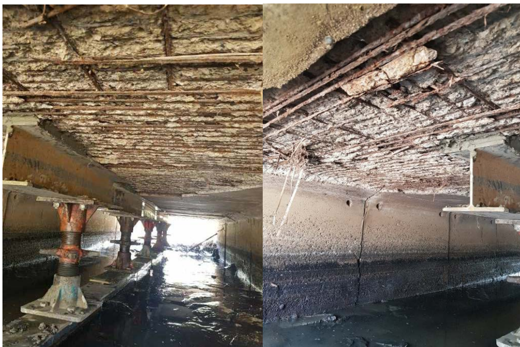
Figure 1: Extent of spalling identified during propping works.
